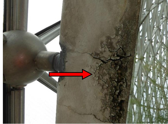
Figure 19. View of cracked and peeling coating on precast member
