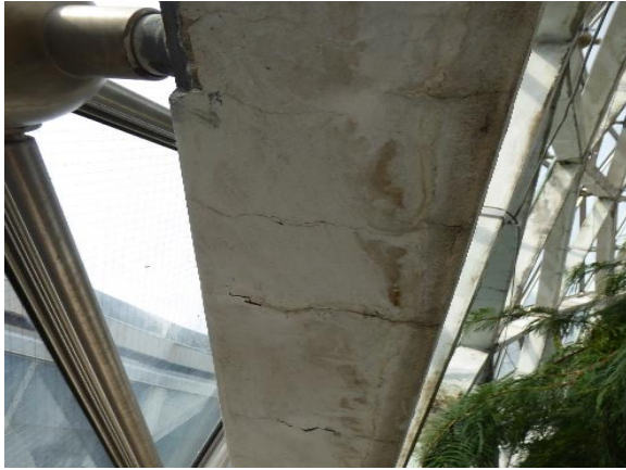
Figure 18. Transverse cracks on precast member
