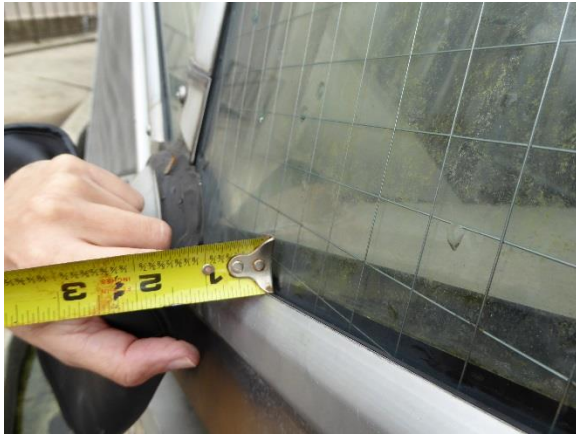
Figure 22. Glazing material at pressure cap on glass cladding
