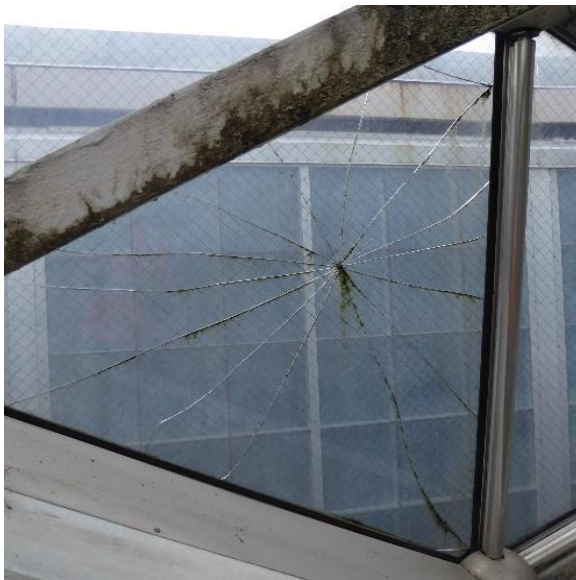
Figure 20. Cracked glass, likely from impact
