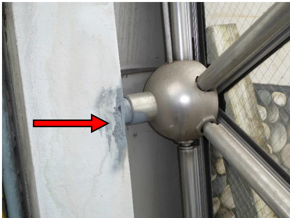
Figure 14. Removed spall at connection location. Note: connection is painted with blue colored coating.
