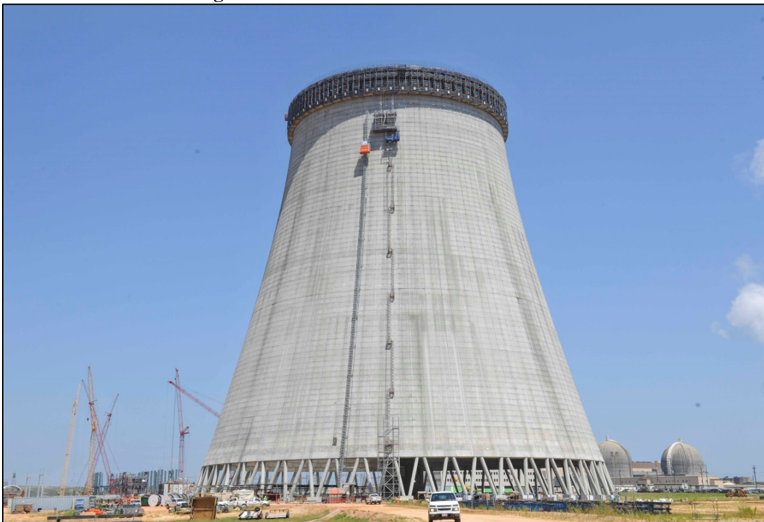
Photo 11 - Unit 3 Cooling Tower Ground View
