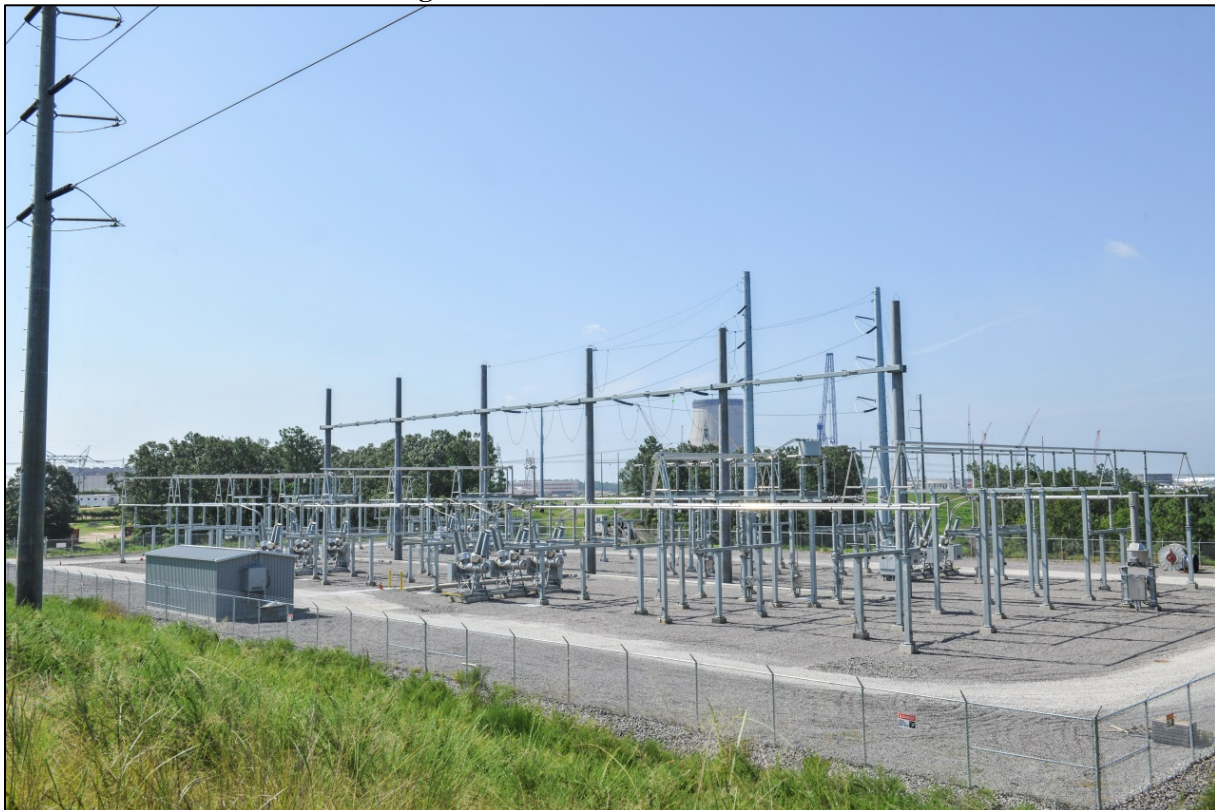
Photo 16 - Unit 3 230kV Switching Station
