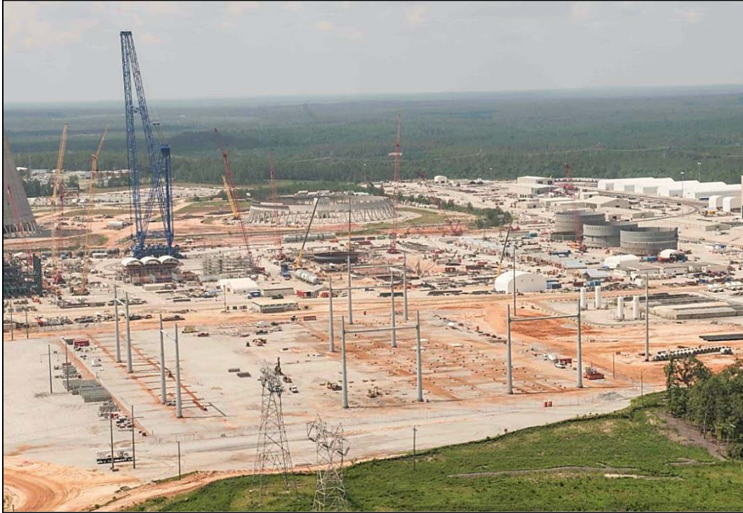
Photo 17 - Unit 4 500kV Switchyard
