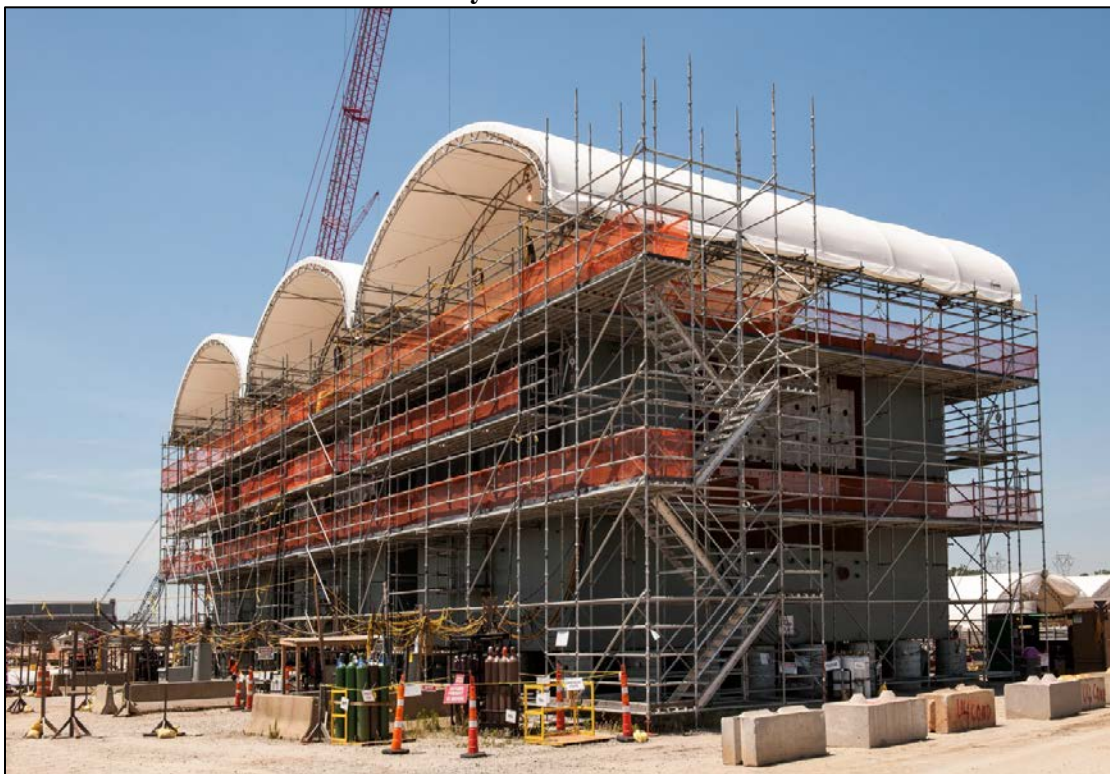
Photo 15 - Unit 4 Condenser Assembly
