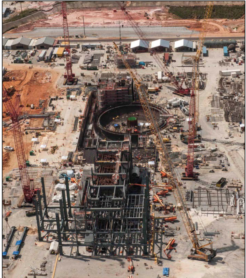
Photo 1 - Unit 3 Nuclear Island and Turbine Island
