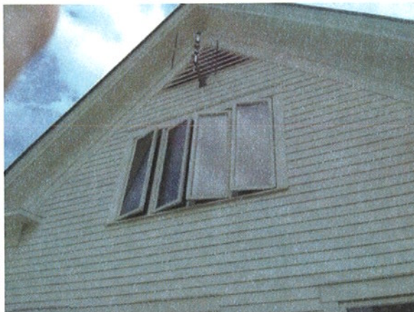
2 nd Floor Bedroom – Partially Open Windows
