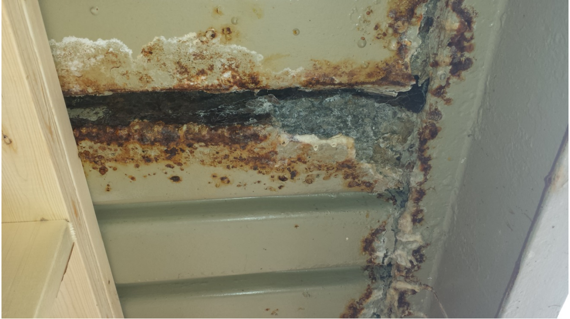
Photo 3: Deterioration at Front Edge of Remaining Walkway
