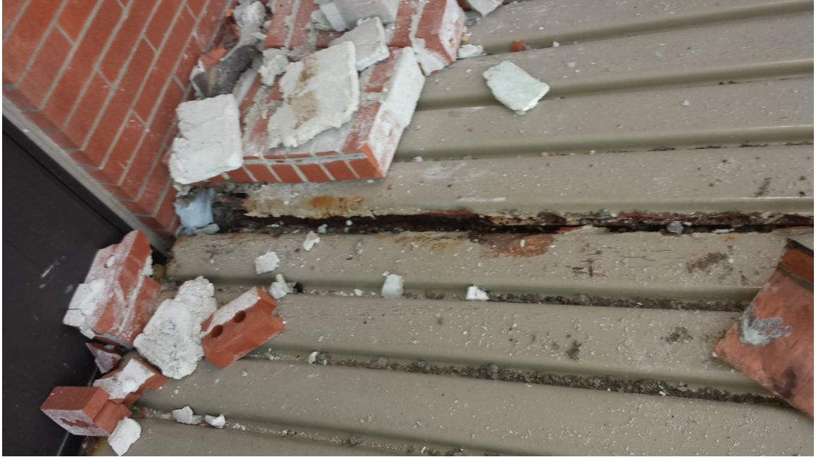
Photo 1: Longitudinal Corrosion and Crack in Metal Deck
