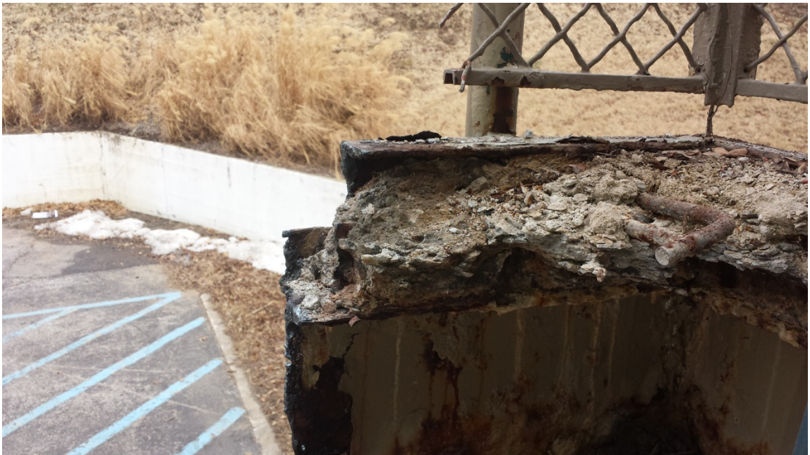
Photo 4: Concrete Shear Failure at Front Edge
