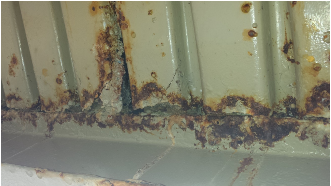
Photo 2: Deterioration at Front Edge of Remaining Walkway
